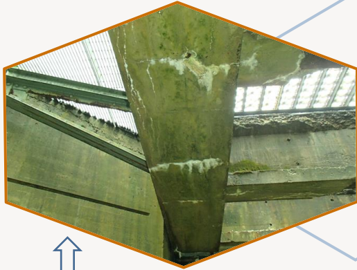
Photo 23 Remaining encasement exhibits fine transverse cracks (spaced 2' to 3') and scattered fine longitudinal cracks, all with light efflorescence stains
