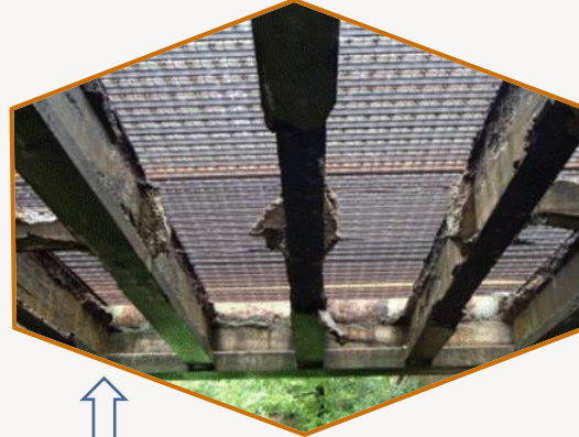
Photo 26 Bays 13W & 14W (4): Concrete completely spalled away/missing with exposed and severely rusted tie rods (est. 70% loss)
