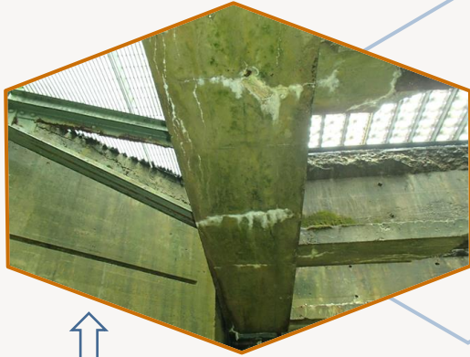
Photo 23 Remaining encasement exhibits fine transverse cracks (spaced 2' to 3') and scattered fine longitudinal cracks, all with light efflorescence stains
