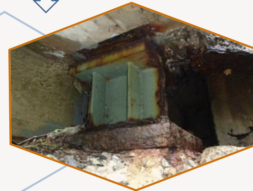
Photo 27 Heavy scaling / disintegration of bridge seat up to bearing masonry plate with minor undermining of southwest corner (< 5%)
